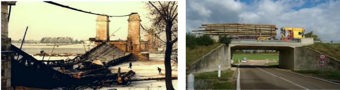
Fig. 2 bridge damage by overload vehicle
